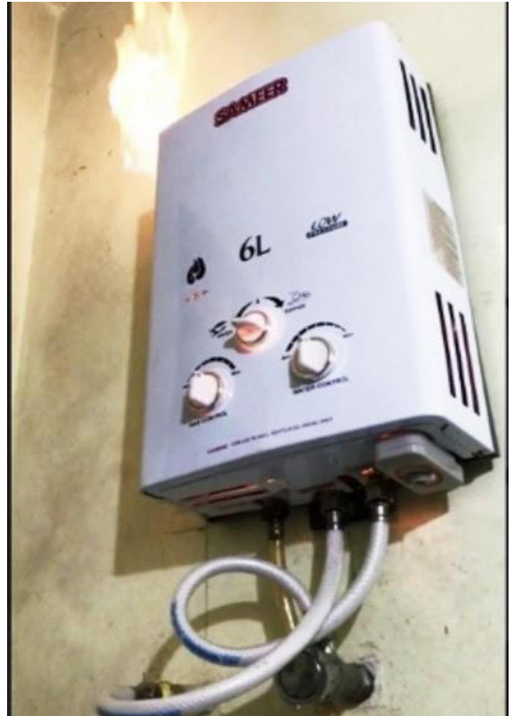
Fig 2. Gas geyser used in bathroom.
